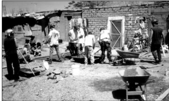
Adults and students prepare cement from tubs and wheel barrels to make the floor of one of the new homes they are building. They already had framed the floor pad and leveled the area earlier in the day. To the left is a cardboard home typical of this section of Juarez. The new home was constructed in front of the recipient family's old home. Photo courtesy of Randy Erickson
