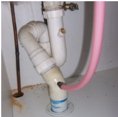
Figure 7 – the exit tubing in position
