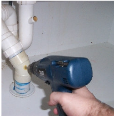
Figure 6 – hole drilled on upper side of pipe, after s-bend
